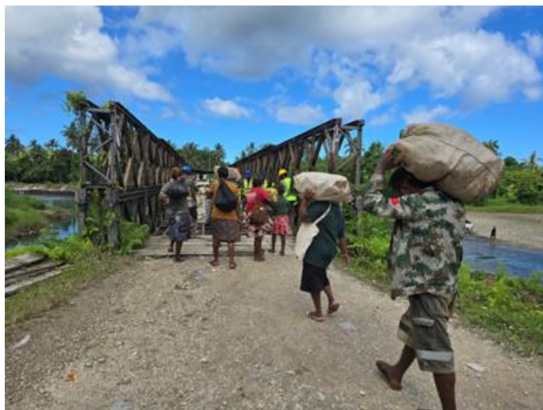
Figure 3: Road users carrying their produces across the collapsed bridge in 2025
