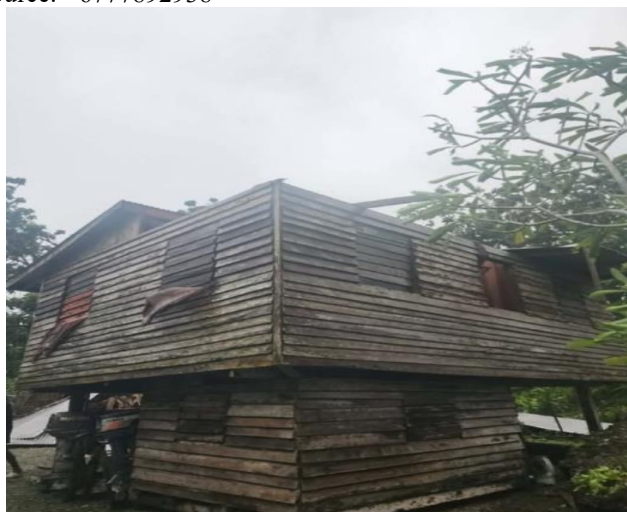
Dwelling houses destroyed by strong winds, Patu. Source: +6777586216
