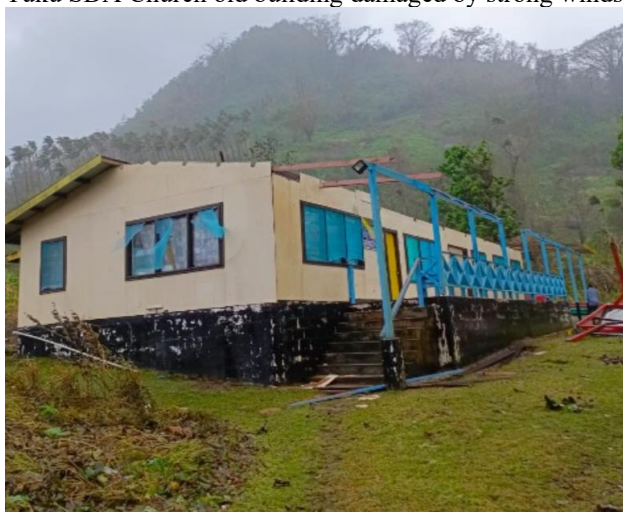
Health clinic destroyed by strong winds, Simbo. Source: Terence Sasapitu
