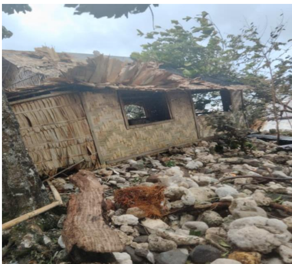
Kitchen damaged by storm surge, Photo Source: Derrick Rooney
