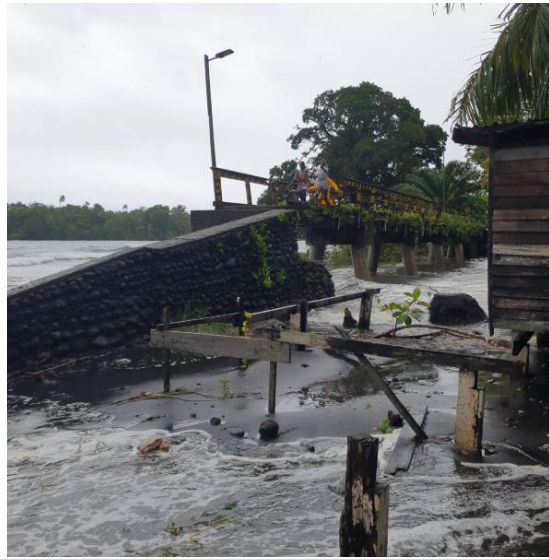
Storm surge destroying footbridge at Ughele Village, Rendova. Source: +6777657504
