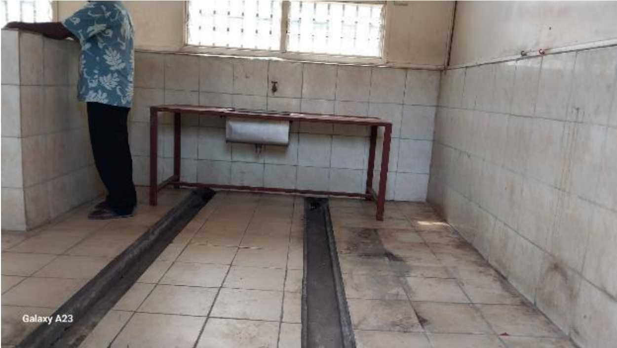
Plate 3: Deteriorated interior of the Slaughter house.
