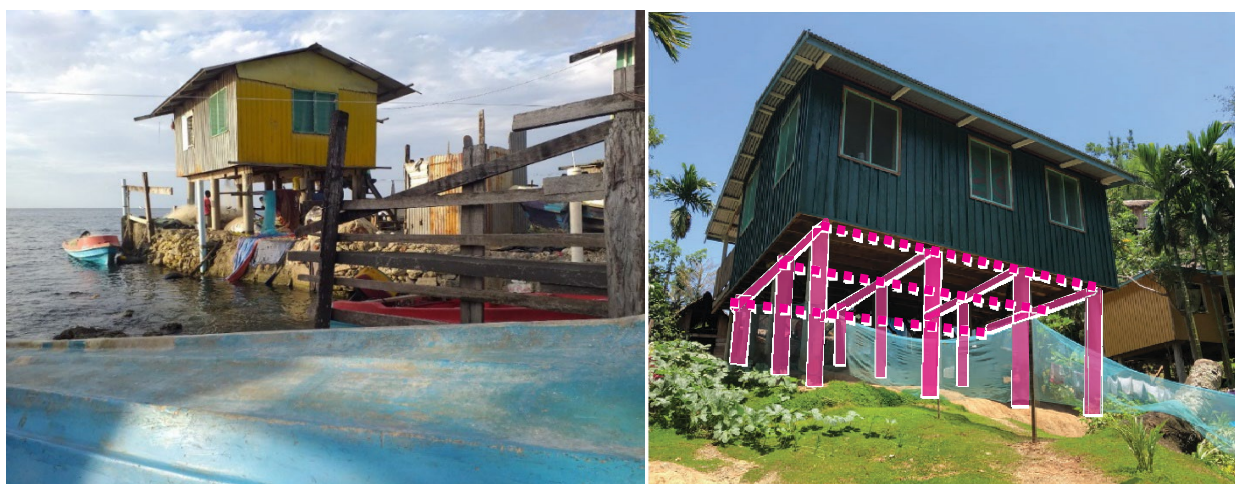
At risk housing: Kukum Fishing Village settlement (L); house on stilts in Wind Valley with dotted lines showing where strengthening is possible (R).
