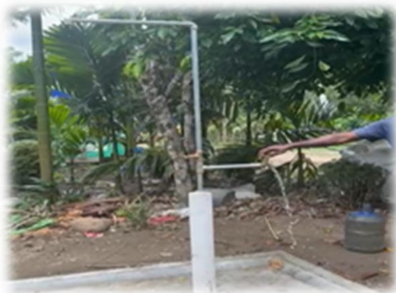
Figure 9: Gravity-Fed Water System Serving Tina River Communities
